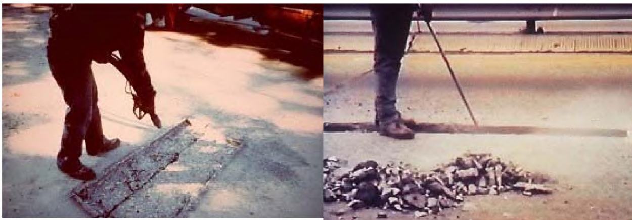
Figure 5. Left: Sand Blasting of Repair Areas. Right: Airblow to Remove Dust and Debris.
